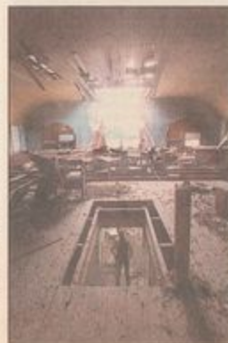
The old school has broken windows and the roof collapsed last June. Glass shards cover the floor and termites have found a home in the rundown building.
